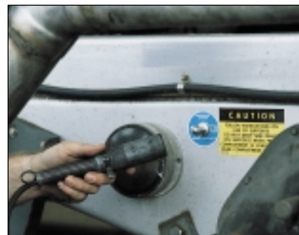
One connection for overfill prevention and earthing
